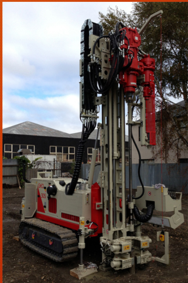
A TONE EP26 SONIC HEAD MOUNTED ON A DRILLTECHNIQUES SOLD AND SERVICED COMACCHIO GEO 305 TRACKED RIG OWNED BY LANDTEST
