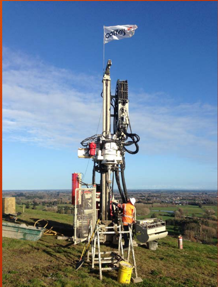
THE SONIC DRILL CORPORATION 50K HEAD MOUNTED ON A DRILLTECHNIQUES SOLD AND SERVICED COMACCHIO 900P TRACKED RIG OWNED BY COFFEY PTY LTD IN OPERATION IN NEW ZEALAND
